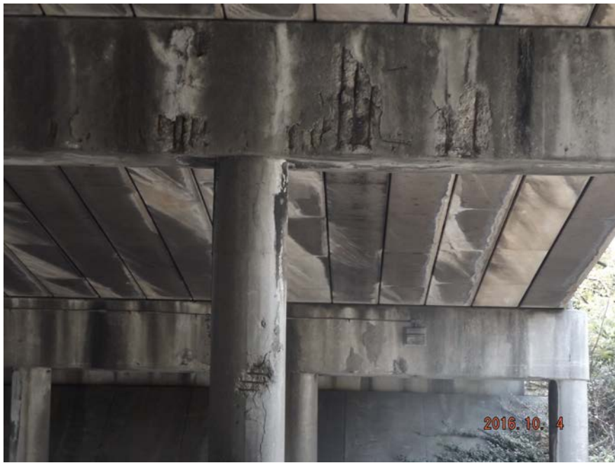
BENT 2 - CAP AND COLUMN B - REBAR SPLLS/DLAMS
