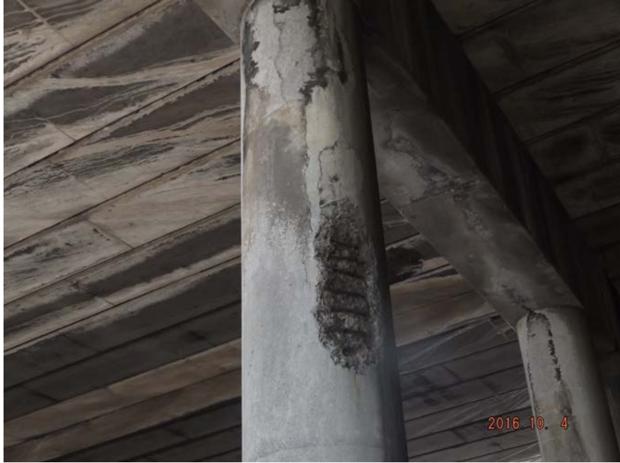
BENT 3 - COLUMN E - LARGE REBAR SPALL
