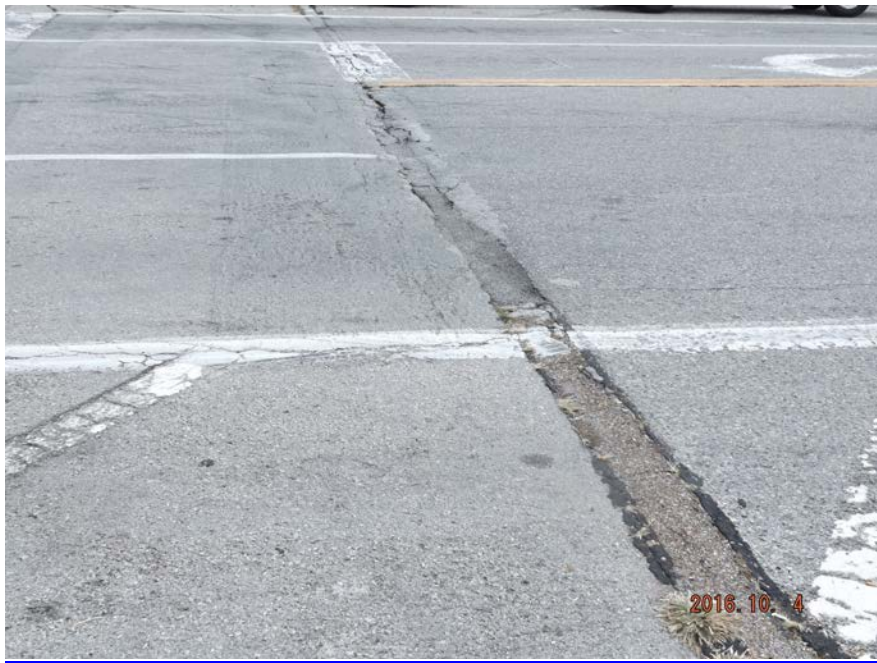
APPROACH 2 - BROKEN - UNEVEN
